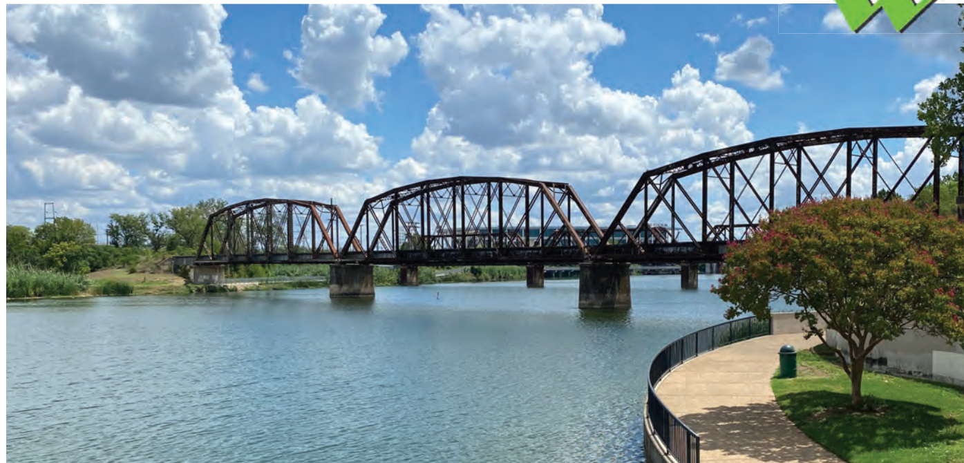
Waco will need to commission a professional engineering report to determine the structural integrity of the Cotton Belt railroad trestle and the span’s suitability for bicycle and pedestrian use.
