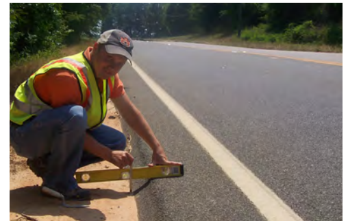
Example of the SafetyEdge SM after backfill material settles or erodes. Source: FHWA
